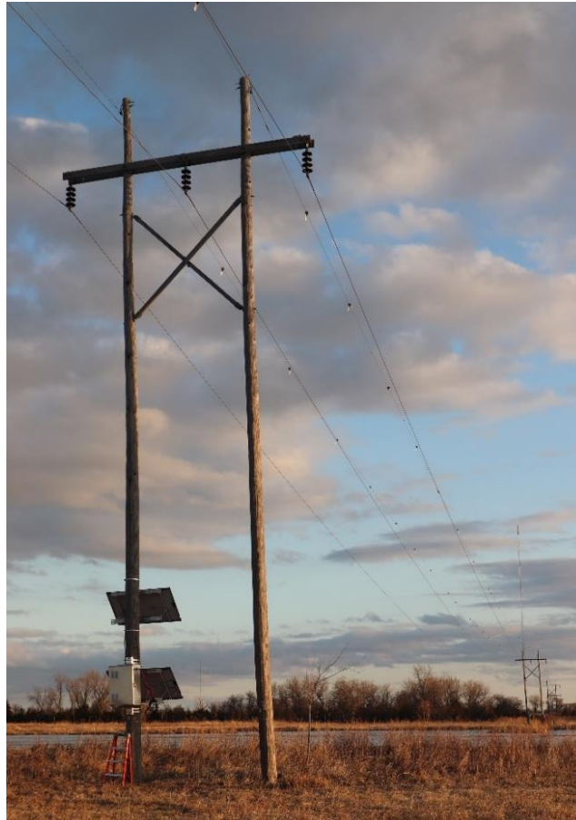
Figure 1. Avian Collision Avoidance System (ACAS) unit mounted on the H-frame structure of a power line crossing the Platte River at Rowe Sanctuary.
