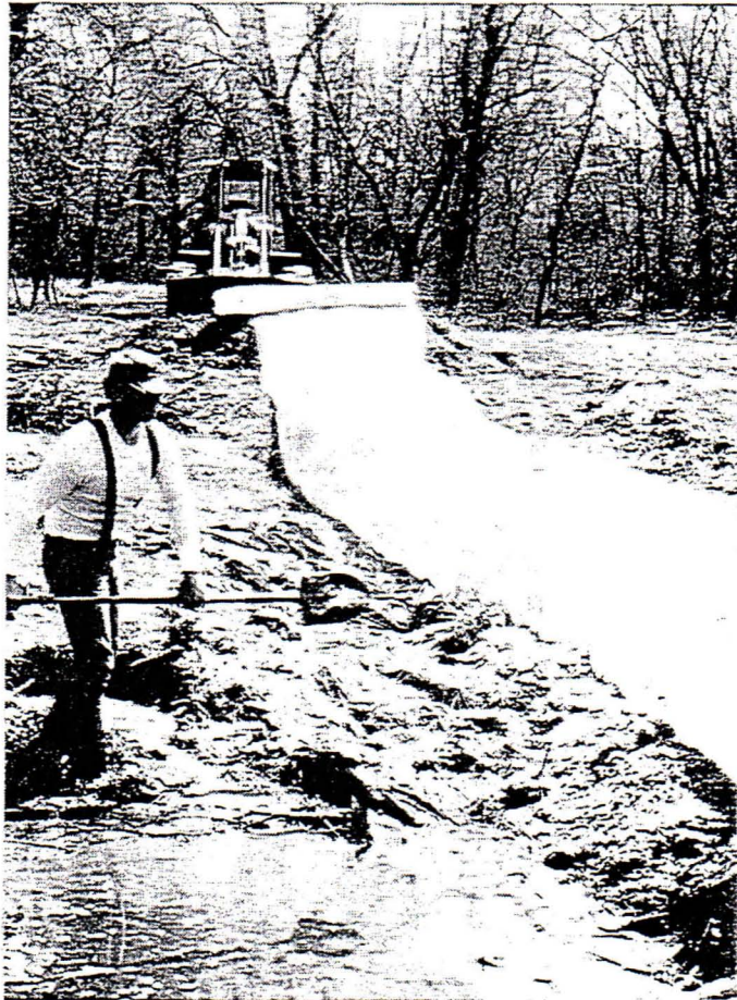
Figure 7. Construction of one of the tube dams across the narrow branch channel of the Platte River. Water seepage below the dams can be seen in each photo.
