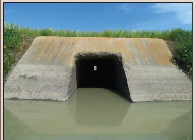
FIG. 2. The 1.8 m x 1.8 m box culvert 89 m long through which Thamnophis gigas #1461 likely passed. The culvert is located 1.2 km south of the east-west canal in which the individual was captured.
